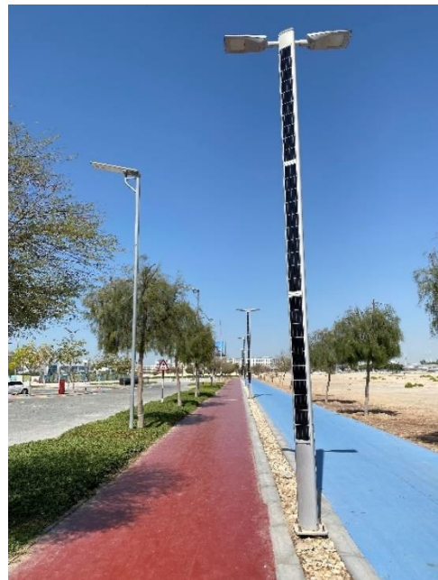
Figure 8. Solar-powered LEDs at Masdar city.
