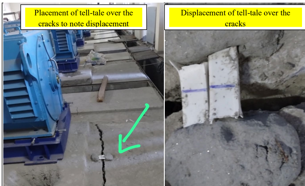
Figure 6. Position of telltale before and after near machine foundation
